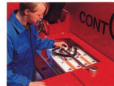
The batteries are well placed to allow easy access and maintenance.
